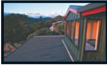
WEATHERED NO CORROSION
